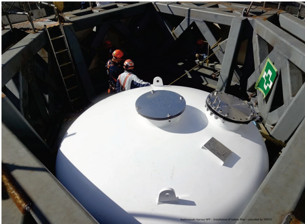
Installation of Iodine filters in Kashiwazaki-Kariwa NPP, ABWR, Japan, Copyright Tokyo Electric Power Company.
