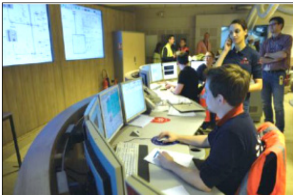
Flamanville 3 – EPR, France, Commissioning supervision in the control room, June 2017 (© EDF All rights reserved. Aménagement Flamanville 3, Communication).
