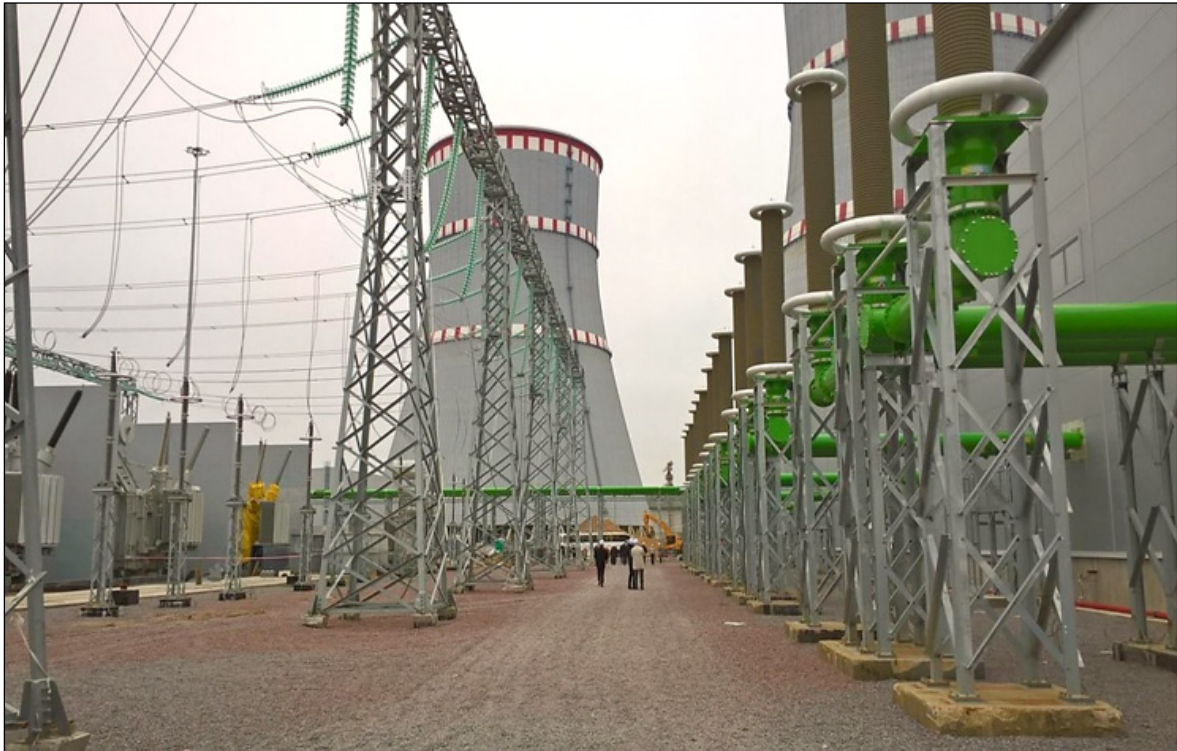
Leningrad 2 – Application of voltage for in-house needs, VVER, Russia, 2017 (Provided by Rostekhnadzor).
