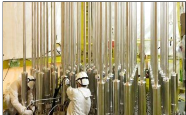
Flamanville 3 – EPR, France, Equipment yard of the vessel head completed: CRDM, June 2017 (© EDF All rights reserved. Aménagement Flamanville 3, Communication).
