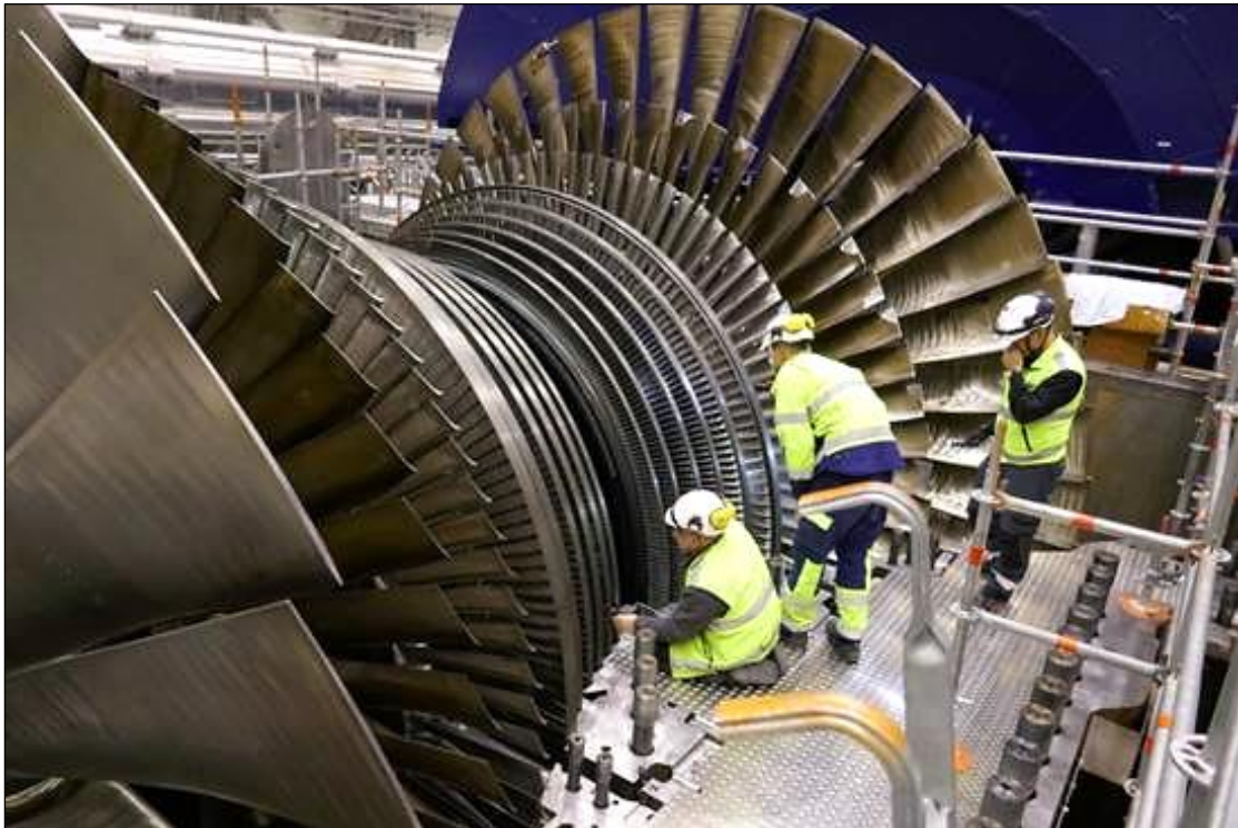
Olkiluoto 3 – EPR, Finland, Turbine island being prepared for hot functional tests May 2017(Provided by STUK).
