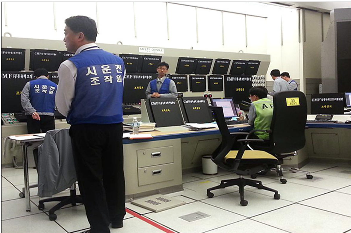
Shin-Kori Unit 3 – Inside Control Room, APR1400, Korea, 2017 (Provided by KINS).
