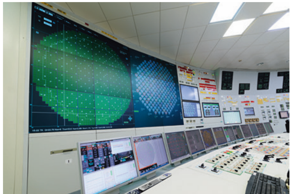
Control room. Shutterstock, Nordroden
