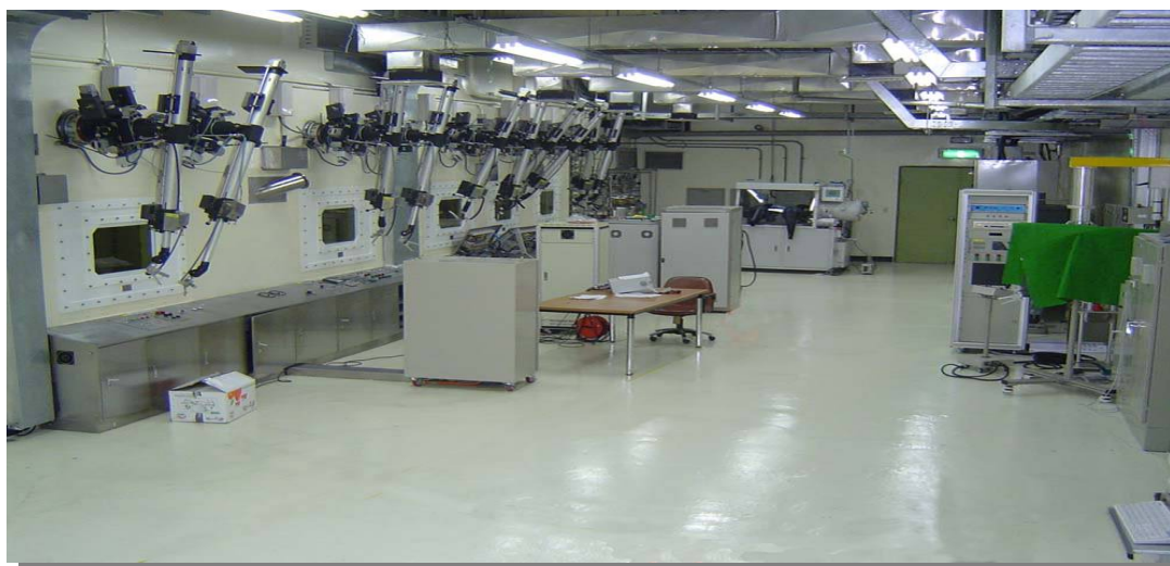
Figure 5.5: Overview of the Advanced Conditioning Process Facility (ACPF)
