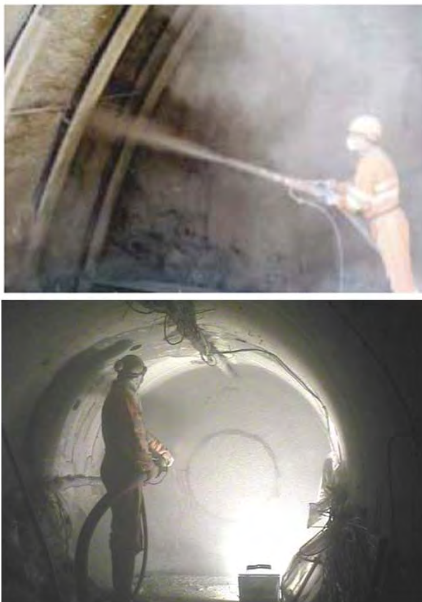
Figure 1: Trials of the use of low pH cements for rock support (top) and tunnel plugs (bottom)
