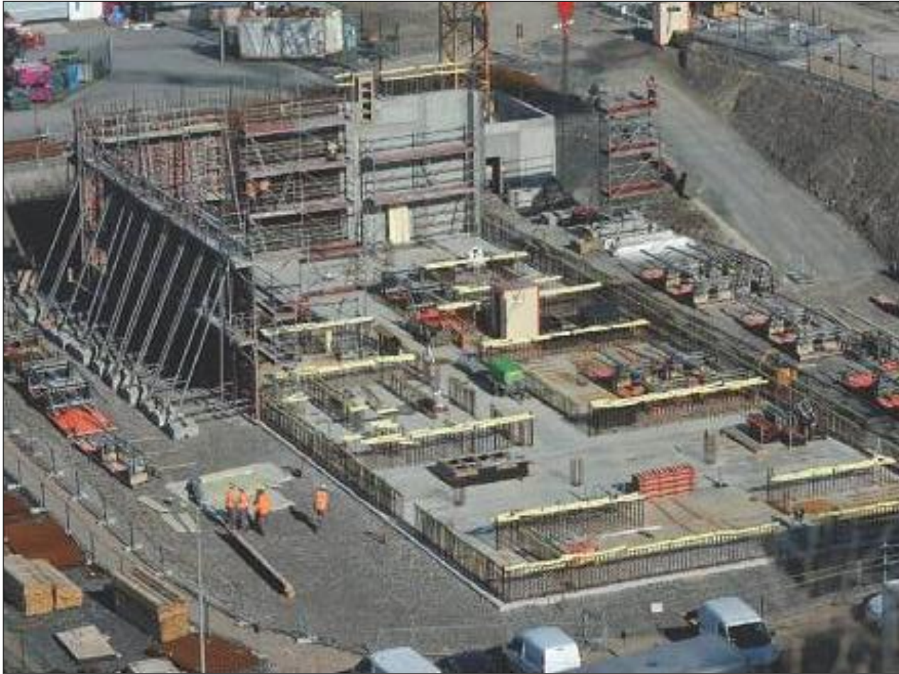
Erection of the new Emergency Control Centre in the Flamanville NPP (Nov. 2014)
