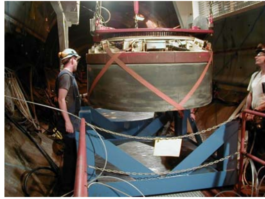
Bentonite buffer ring emplacement (Sweden)
