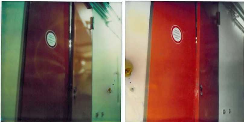
Figure 0-4: Photographs of the damaged fire door from outside the room
