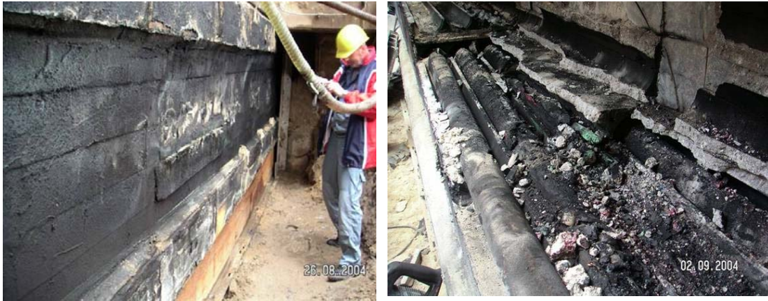
Figure 0-1: Photos of the cable damage; left: location of the damaged cable, right: damage by the cable fire/evaporation
