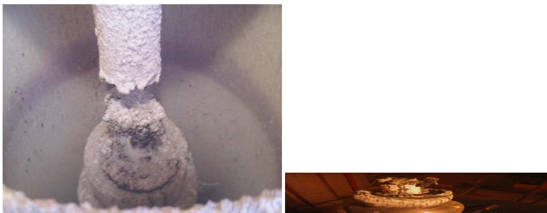
Figure 0-11: Photos of the bushing damage
