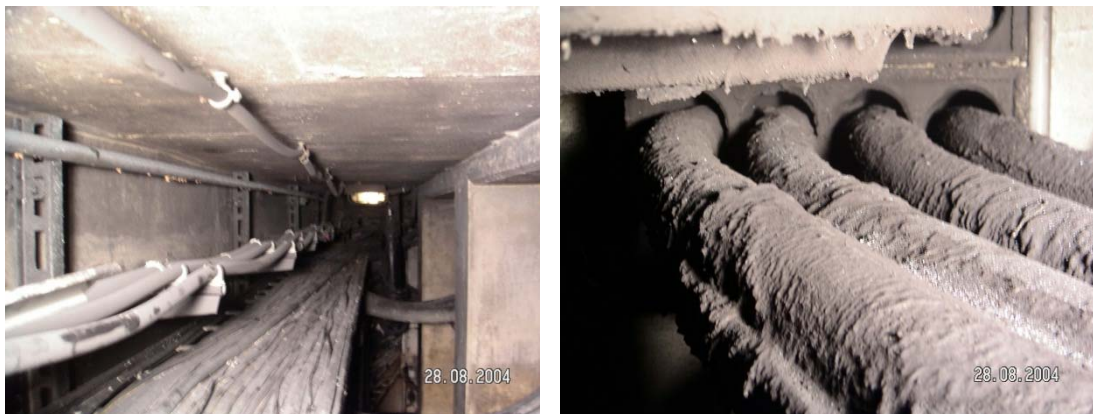
Figure 0-2: Cables with protection by intumescent coating; left: photo of the cable channel, right: photo of the coating
