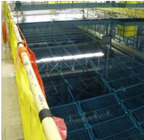
Figure 7: CANDU storage bay with fuel racks.
