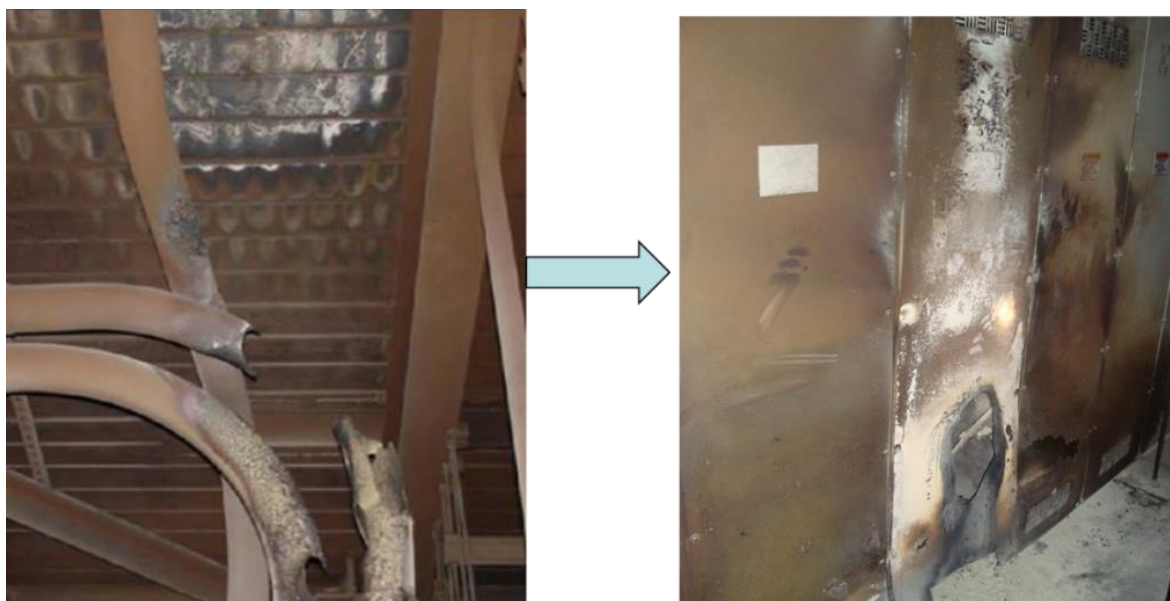
Figure 12. Damage at bus 5 (on the left) and 4
