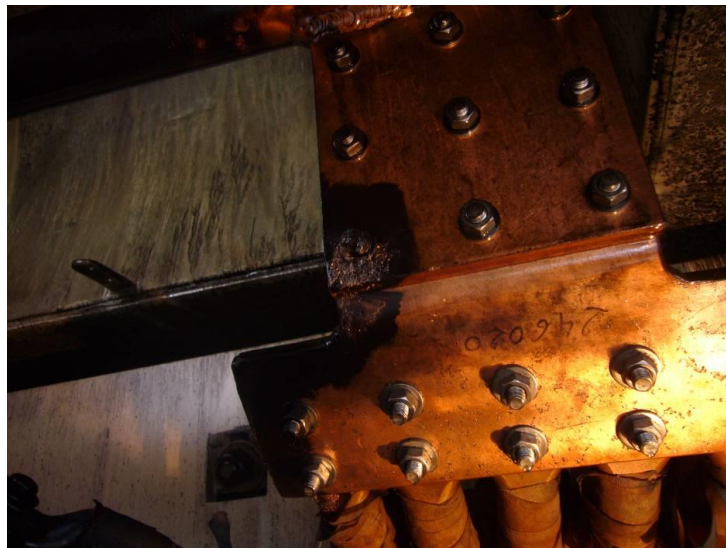
Figure 15. Screws of steel employed to hold the wooden support pad of low voltage bus bar system
