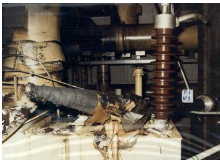
Figure 14. Damage due to fire
