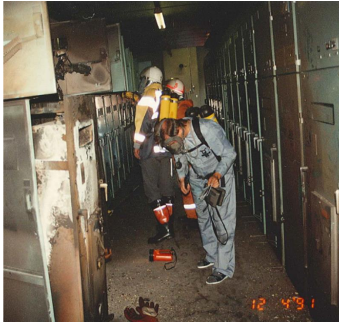
Figure 10. Switchgear room with damaged and undamaged switchgears
