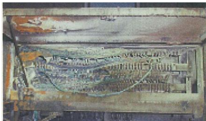
Figure 22. Damage after the event in the control duct
