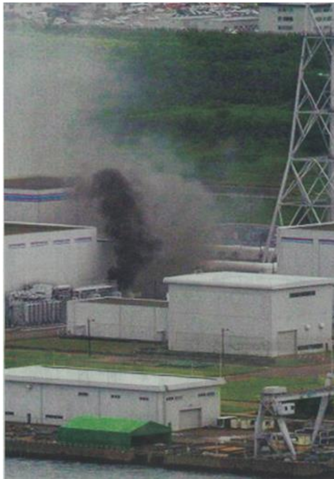
Figure 16. Seismically and HEAF induced fire at a station transformer
