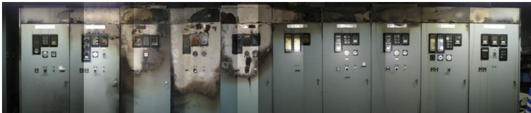
Figure 21. The ten connected cabinets with damage after the event
