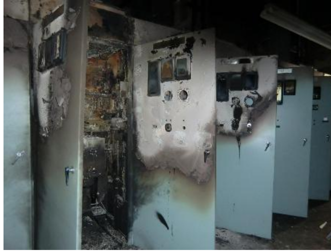
Figure 20. Electric cabinet with the sector on the left where the fire started
