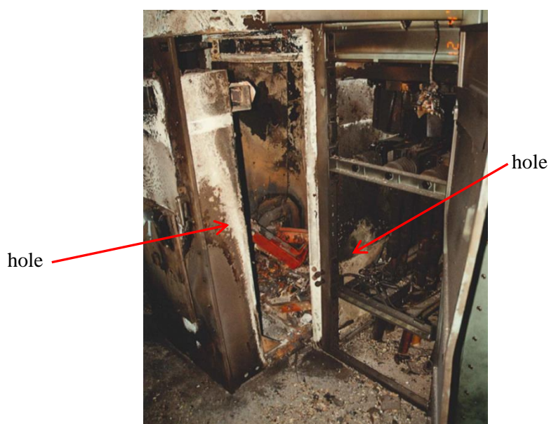
Figure 8. Lower part of the 6 kV cubicles no. 2 and 3 damaged by fire and HEAF
