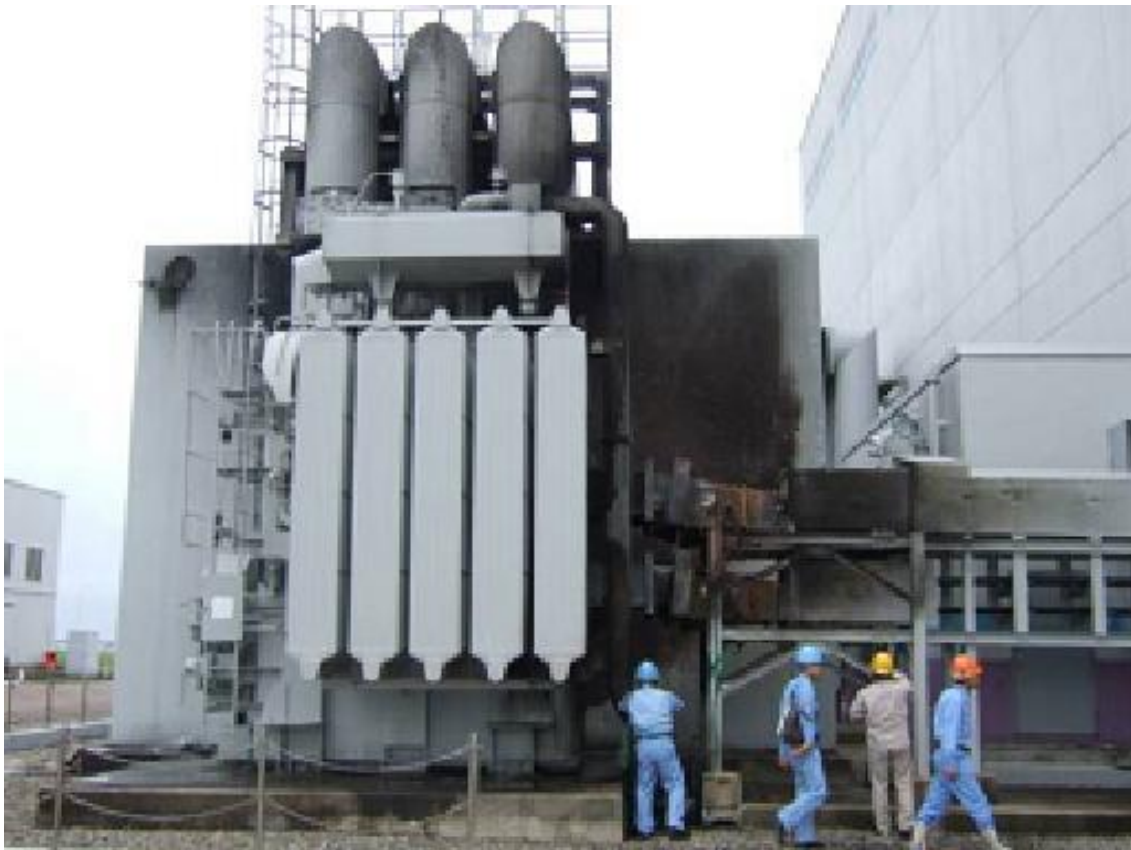
Figure 17. Damaged transformer after the fire
