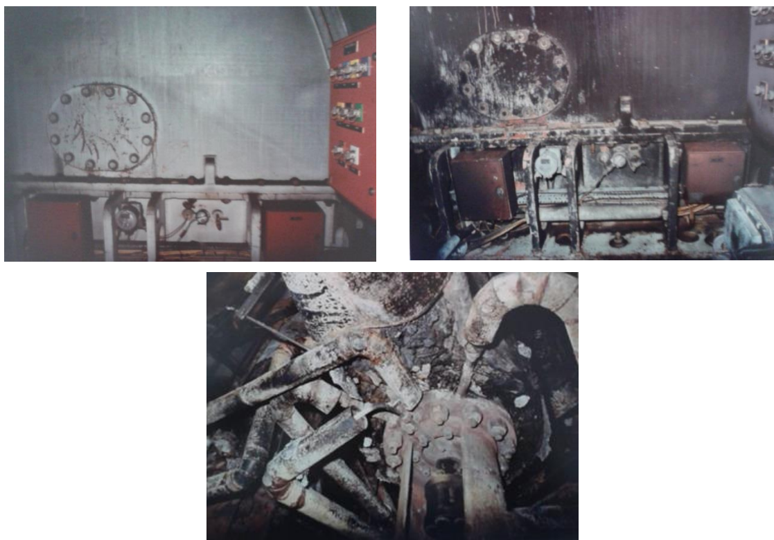
Figure 6. Damages due to the fire in one of the event combinations of fire and consequential fire
