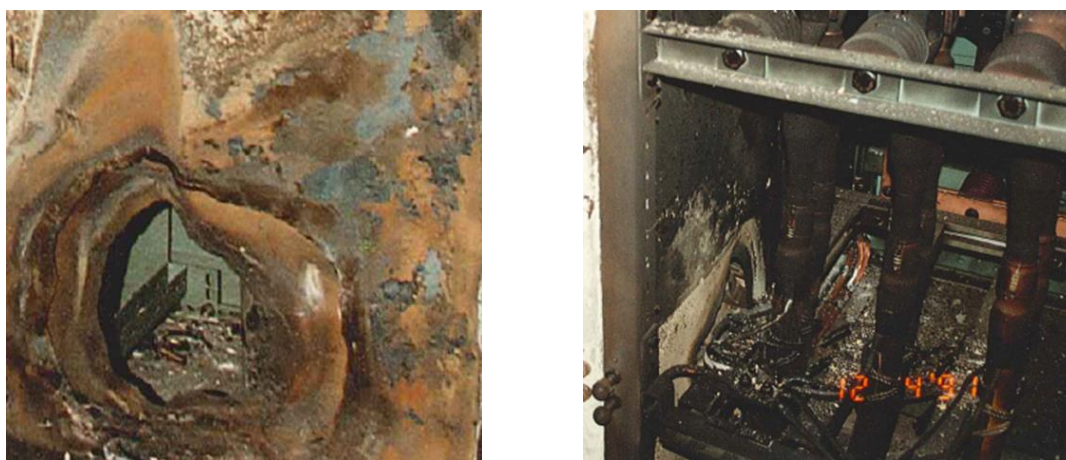
Figure 9. Damage of a fire with consequential HEAF: hole in the wall separating the cubicles no. 1 and 2 (left), the hole in the wall separating the cubicles no. 2 and 3 (right)
