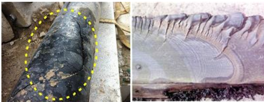
Figure 31: Ruptured Buried HDPE Fire Water Pipe and Cross Section.
