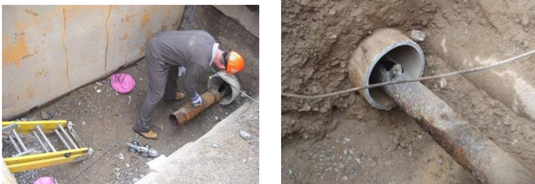
Figure 16: NPS 6 Buried Condensate Discharge Line Exhibiting Corrosion Under Insulation (CUI)
