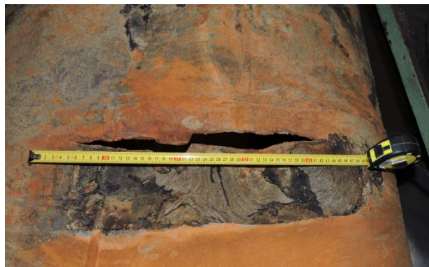
Figure 17: Damage to DN800 ESW Pipe 22
