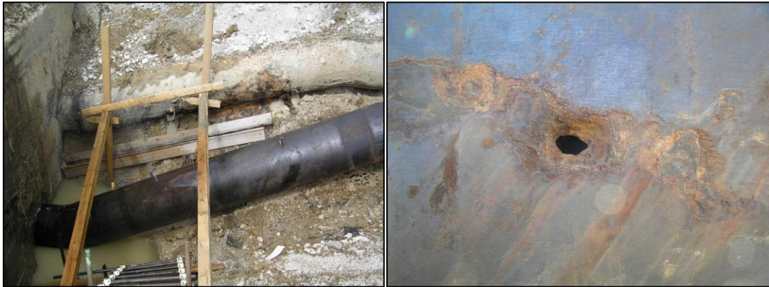
Figure 22: The Leaking on the Return pipe DN800 on the ESW System I Near the ESW Cooling Tower.
