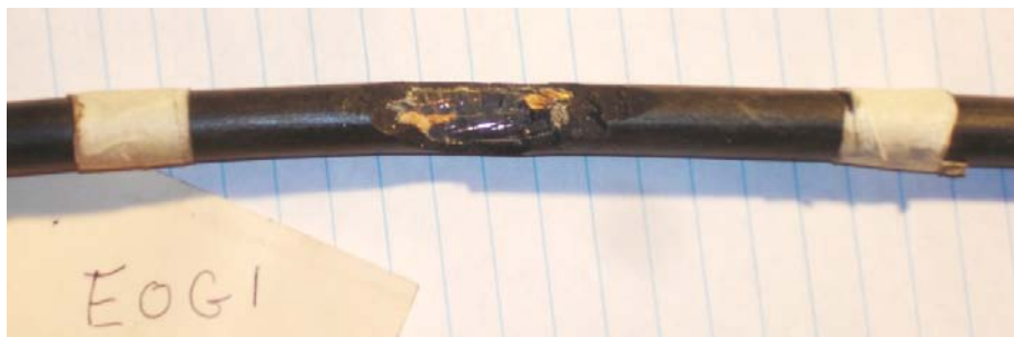
Figure 3.3.9-1: Mechanical damage on a low voltage cable
