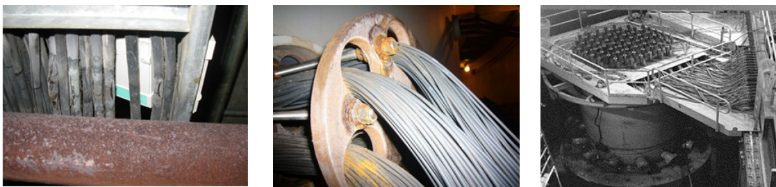
Figure 4.4: Cable exposed to high ambient, mechanical stress (sharp metal edge), and radiation effected cables on reactor head
