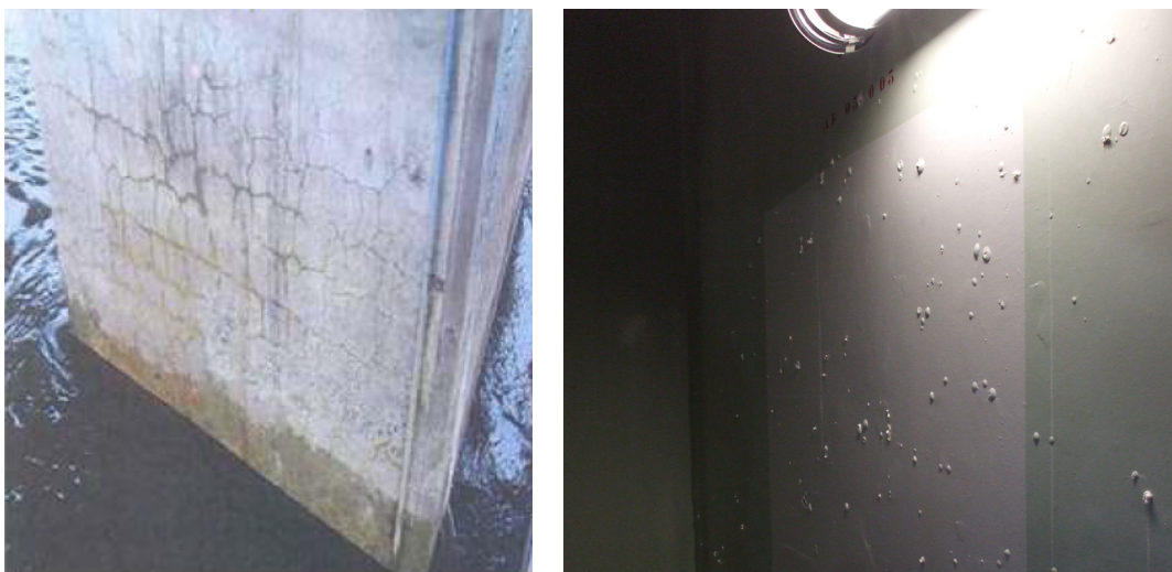
Figure 4.3: Example of pattern cracking and pop-outs of ASR-affected concrete
