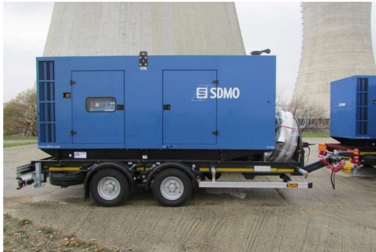
Figure 4. Mobile Diesel Generator 4 x 352 kW (one per unit)
